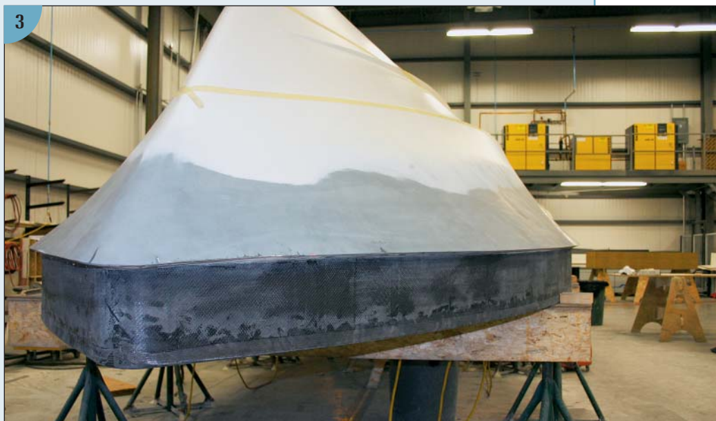
(3) A carbon fiber hull under construction. This entire hull and deck weighs under 600 pounds. With a hull this light, you can use smaller engines, carry less fuel, and achieve a much higher performance.
