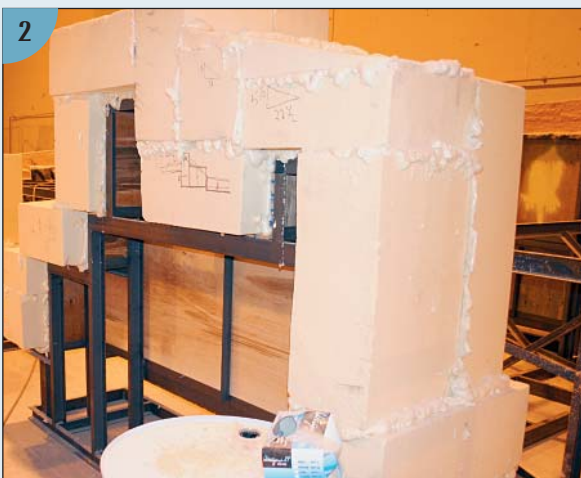
(2) Foam blocks are glued to the armature. Filler foam has been sprayed between the blocks to help glue them together.
