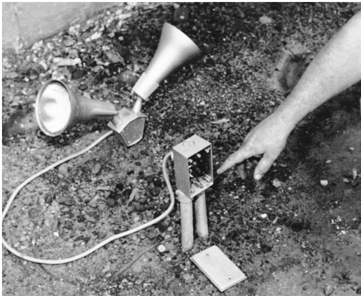
Fig. 400-3. This use of flexible cord to supply an outdoor lampholder assembly can readily be described as a “substitute for fixed wiring”—which is a prohibited use of cord. Here, the lampholders could have been attached to one or more threaded openings on an outlet box. (Sec. 400.8.)
